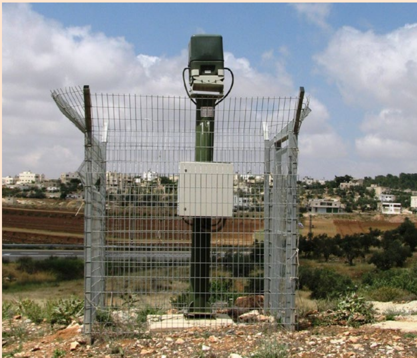
Motorola radar system at the Otniel settlement, May 2011. (Photo: Who Profits)
