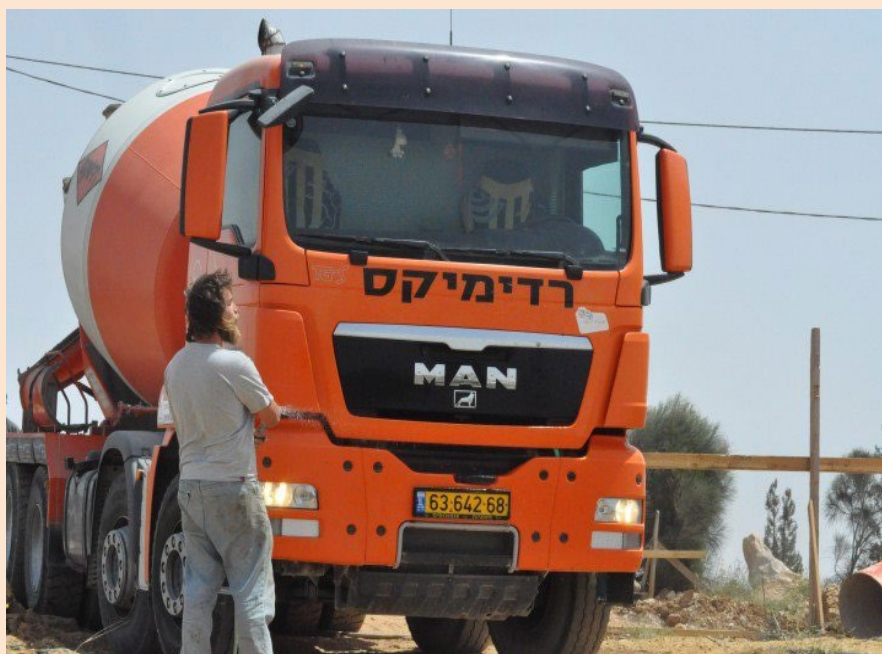
A Readymix truck delivering concrete to the Mitzpe Yair outpost, May 2012. (Photo: Guy Taayush)
